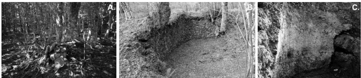
Figure 6.8. A) Hut ( choza , cabaña or txabola ) serving as temporary shelter for many inhabitants of the forest; B) ice house with circular stone structure; C) limekiln with putlog holes.
