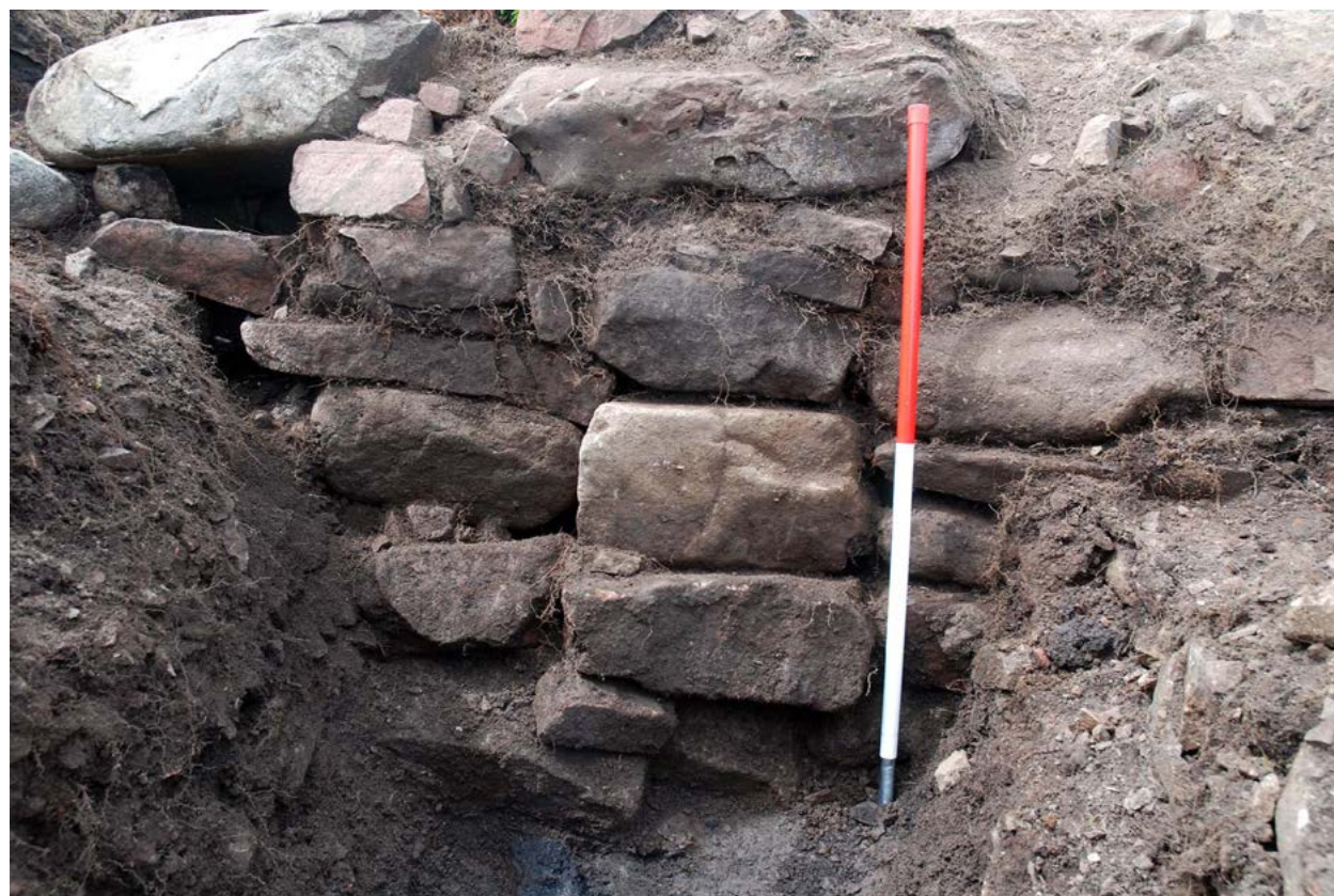
Figure 6.14: The inner face of inner wall in Area A, showing the possible repair in the façade.
