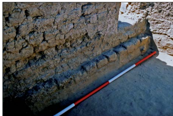
Plate 3.20. The foundation courses of the south wall in Room A1-II – scale bar 2m.
