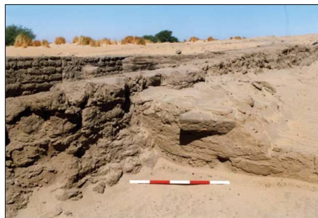
Plate 4.49. The street between Buildings B1 and B2. Successive crusty surfaces designated (BF3)56 against the east wall of Building B1, looking north west. Note the severe damage caused by erosion of the outer face of the wall – scale bar 500mm.
