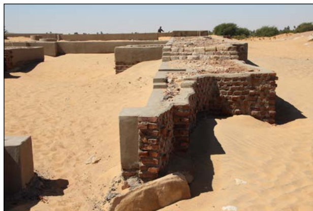
Plate 16.20. Missing section of wall at the north-east corner of the temple indicated by unplastered and irregular brickwork.
