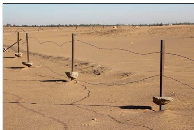
Plate 16.13. Wind erosion removing the ground surface and exposing the concrete into which the fence posts had been set.
