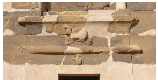
Plate 12.13. The lintels over the doorway into the offering chapel of Pyramid Beg.S.7 in the South Cemetery at Meroe.
