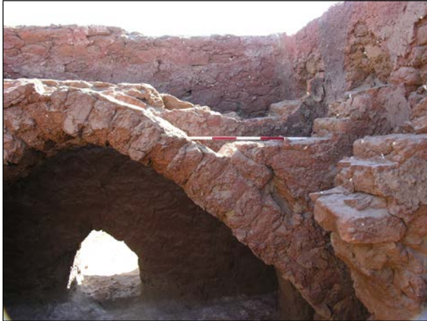
Plate 7.17. Building F7. Cross wall partly preserved to its full height – scale bar 500mm.
