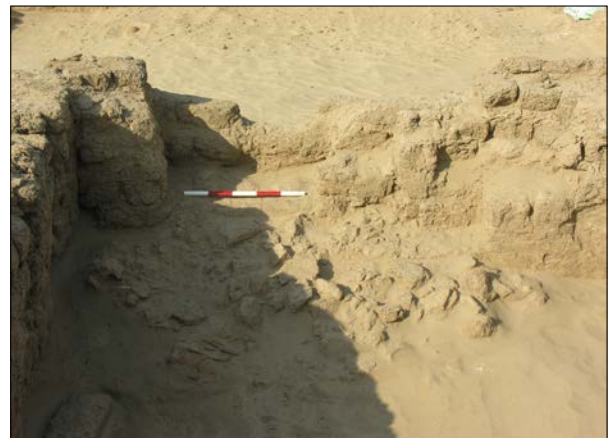
Plate 3.49. Building A2, Room IV, rubble (AD5)48 in the doorway leading to Room III – scale bar 500mm.
