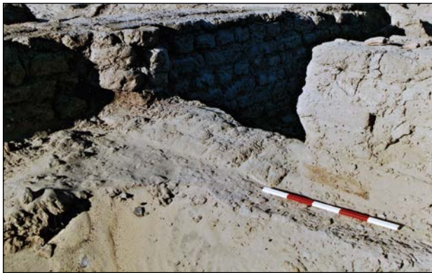
Plate 4.10. Building B12. Doorway with timber threshold between Rooms VII and XVIII, looking south west – scale bar 500mm.
