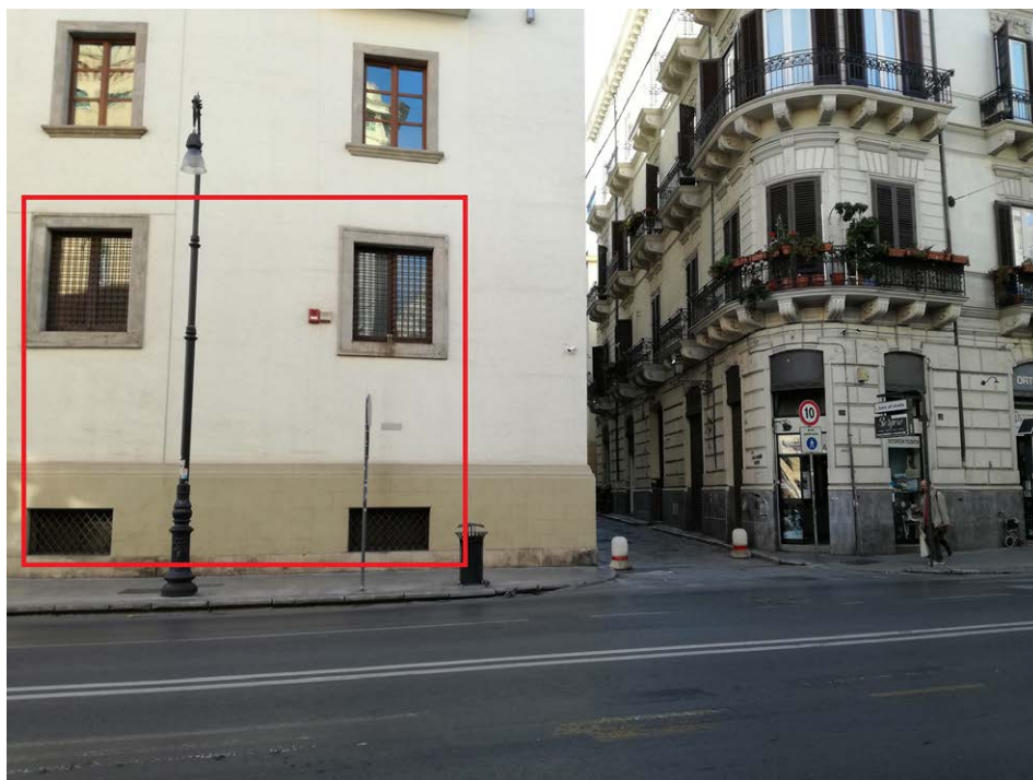
Figure 4.17: The breach in the museum's façade on the Via Roma (source: author).
