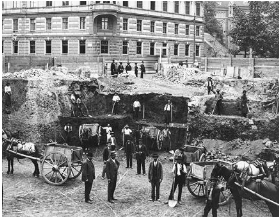
57. Excavations started in Vienna during the major construction work removing the former city defences in the second half of the 19th century
